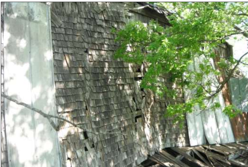
Figure 6-46. Resource 2—Collapsed Porch Roof on Southern (Front) Façade of House (Facing Northeast)
