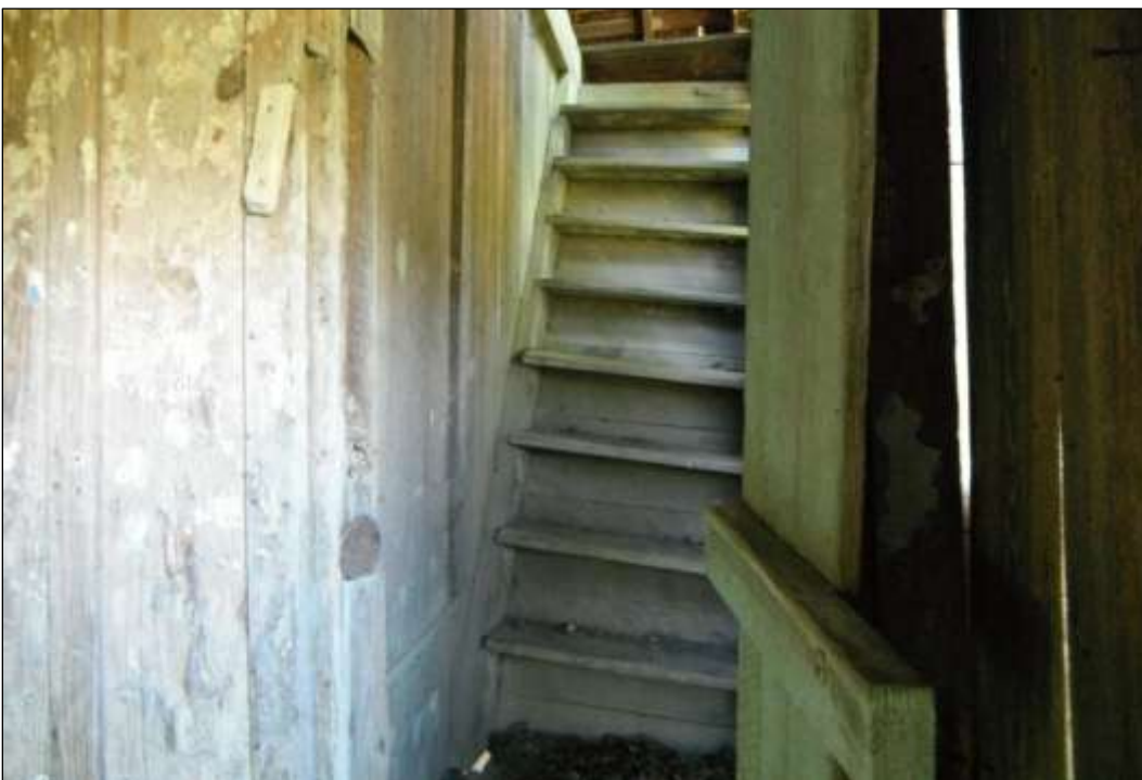
Figure 6-50. Resource 2—View of Interior Enclosed Stairs Leading to Sleeping Loft (Facing South)
