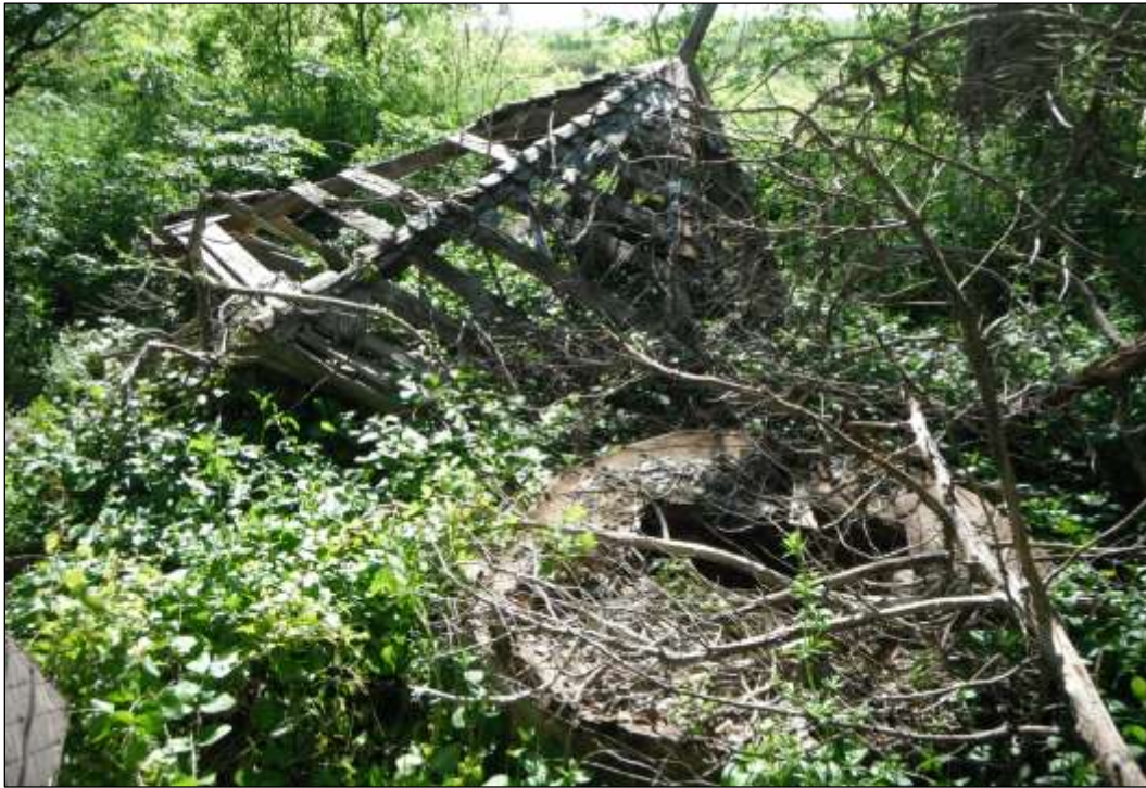
Figure 6-23. View of Collapsed Wooden Gazebo and Covered Limestone Well Adjacent to Main House on Site 41TV2518 (Facing South)
