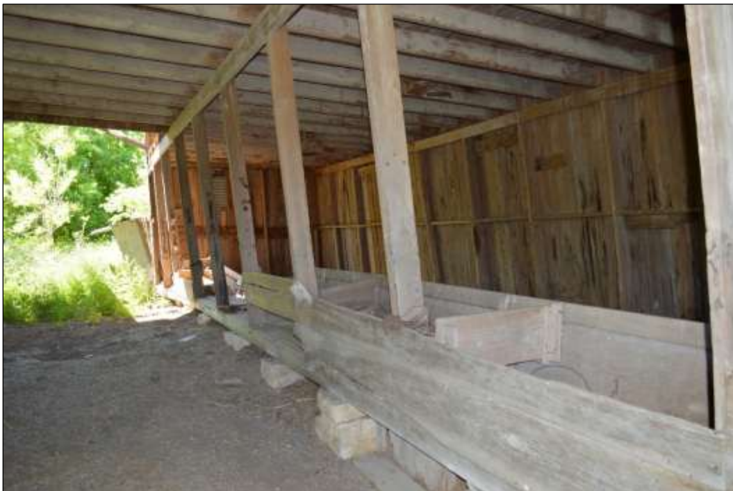
Figure 6-31. Resource 1C—Open Stalls and Feeding Trough along Western Side of Barn Interior (Facing Southwest)
