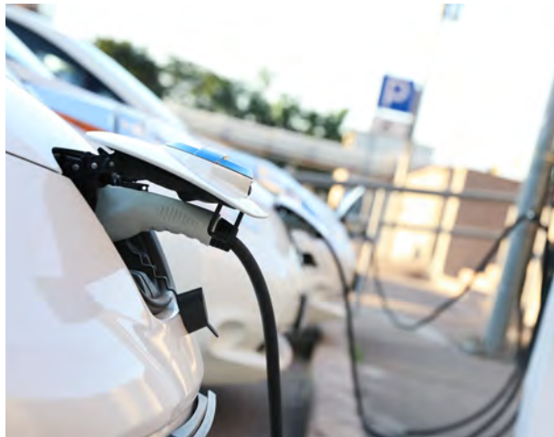
EV charging stations
