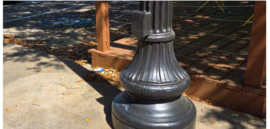
Fluted light pole bases with power receptacles
