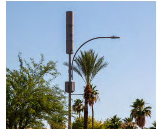
5G antenna on light pole
