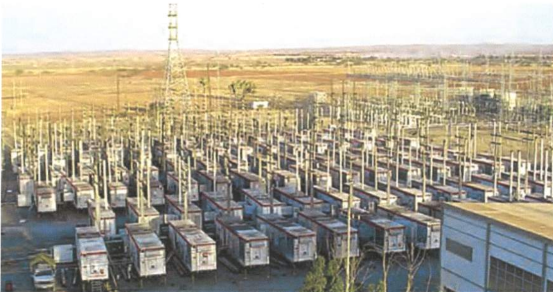
Above: (100) containerized 2.0 MW generators - Utility paralleled & running continuous 24/7 duty cycle
