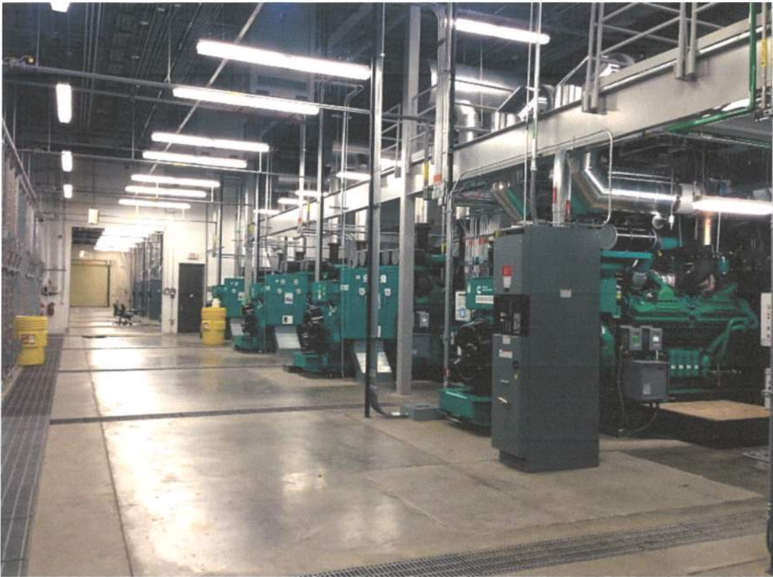
Above: Genset building with (12) 2.25MW generators & EPA certified Tier IV after treatment equipment
