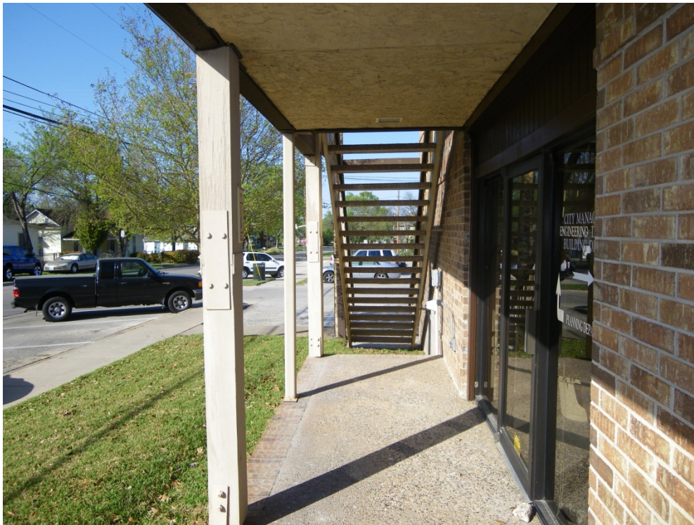
3. West side of Suite 300 –ADA non-compliant protruding object
