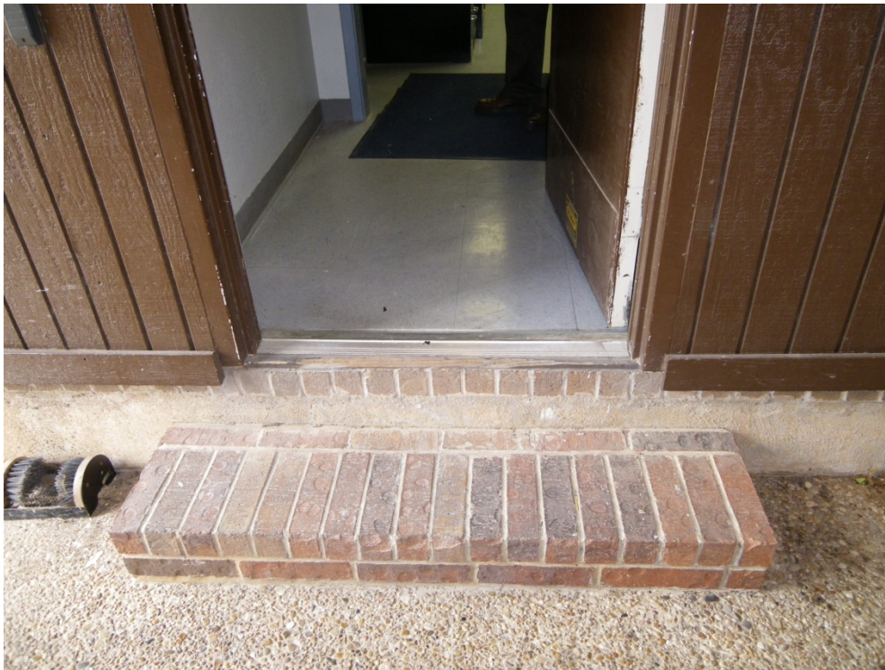
5. Typical ADA non-compliant accessible staff entrance/exit
