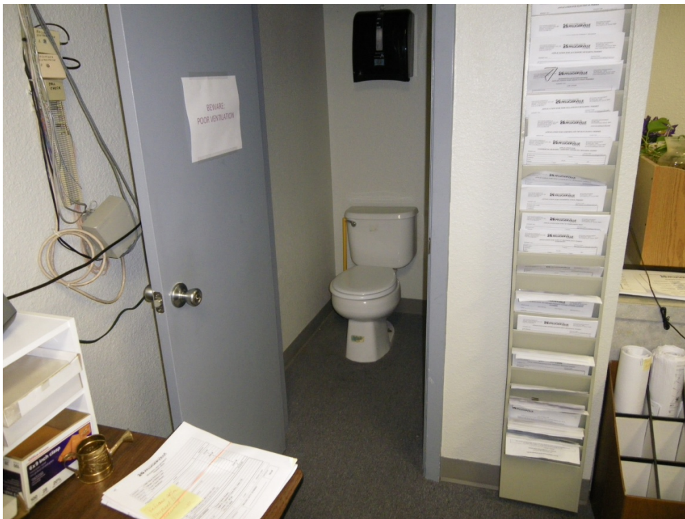
8. ADA non-compliant restroom – Building 200
