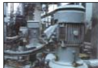
Duty Master XT Vertical Motors drive in-line process pumps in petroleum refining operation.
