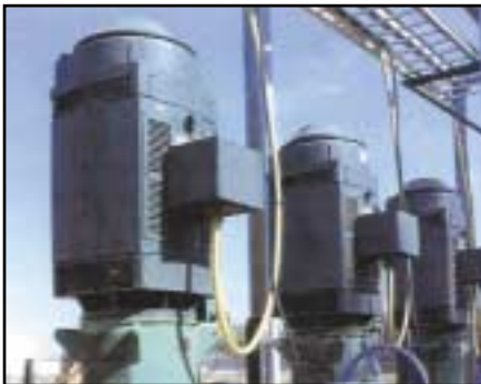
A clear water feed pump in a paper processing operation is driven by a Weather-Protected NEMA type 1 Duty Master Vertical Motor.
