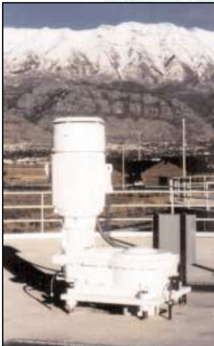
One of eight Reliance vertical P-Base motors in use at a wastewater treatment plant.
