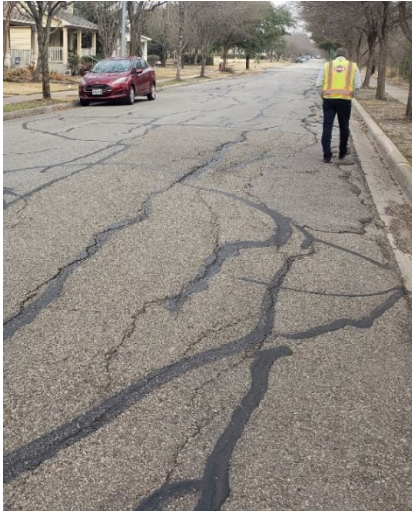
Wide Longitudinal Cracks, Differential Vertical Movements on Pavement and Curb & Gutter, Exposed Base
