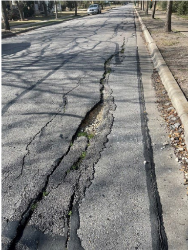
Wide Longitudinal Cracks, Differential Vertical Movements
