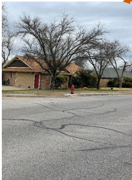
Longitudinal and Transverse Cracks
