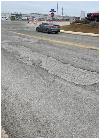
Alligator Cracks, Transverse Cracks, Loss of Bond between Asphalt Layers
