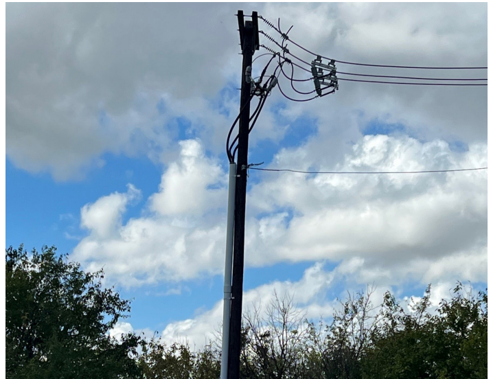
Pole with Riser
