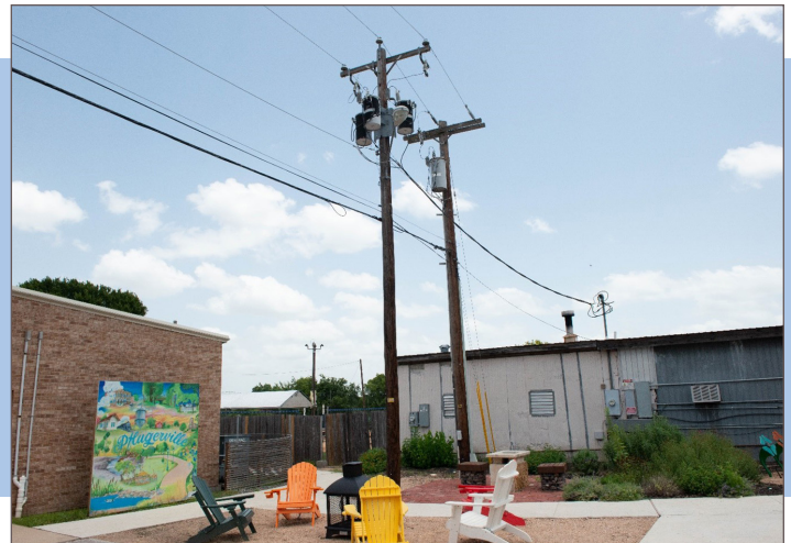
Overhead utility lines traversing the City Hall site and the Best Little Plaza in Texas
