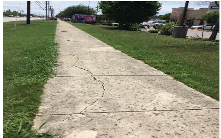
Figure 3-14: Cracked Uneven Sidewalks along FM 685
