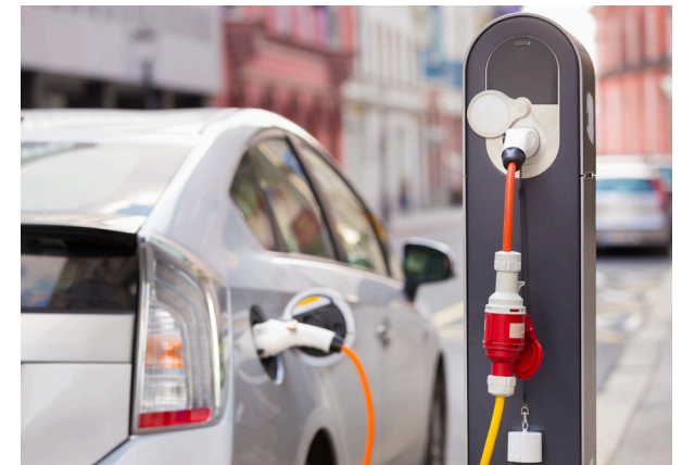
Charging station in parking lot
