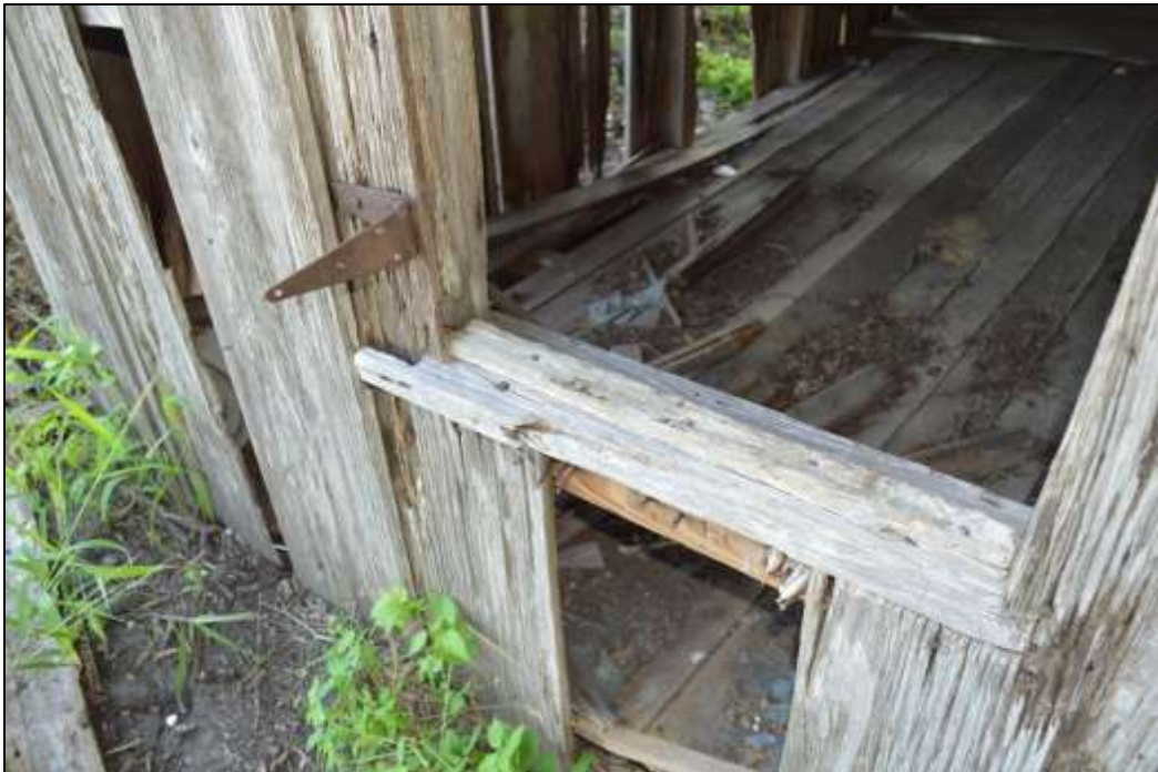
22. Window sills, jambs, and rail guards on west façade of house
