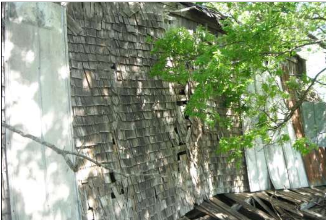
Figure 10. Collapsed Porch Roof on Southern (Front) Façade of House (Facing Northeast)
