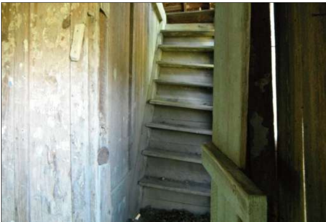
Figure 12. View of Interior Enclosed Stairs Leading to Seeping Loft (Facing South)
