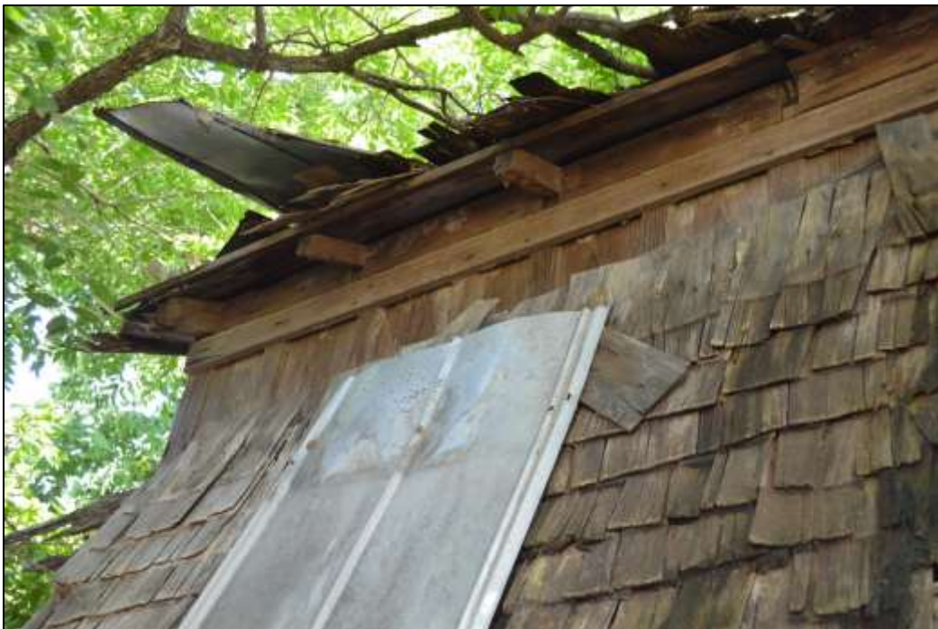
32. Roof construction showing rafters where porch has collapsed
