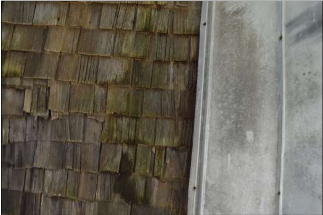
25. Detail of roofing material on collapsed porch roof
