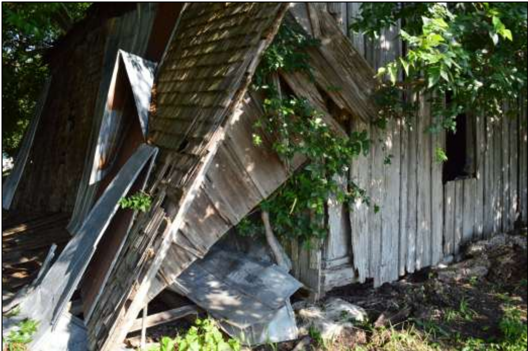
26. Collapsed porch roof at southeast façade
