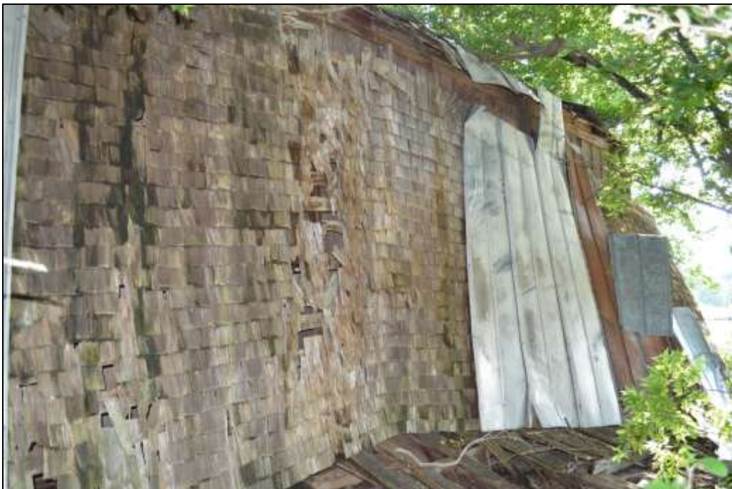
24. Collapsed porch roof on south façade of house
