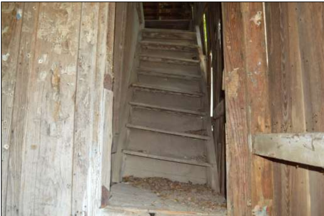
40. Looking up from bottom of stairwell through door from the northwest room
