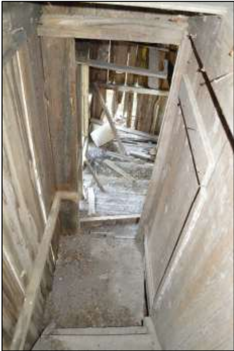
37. Looking down from top of stairwell; note original door on the right
