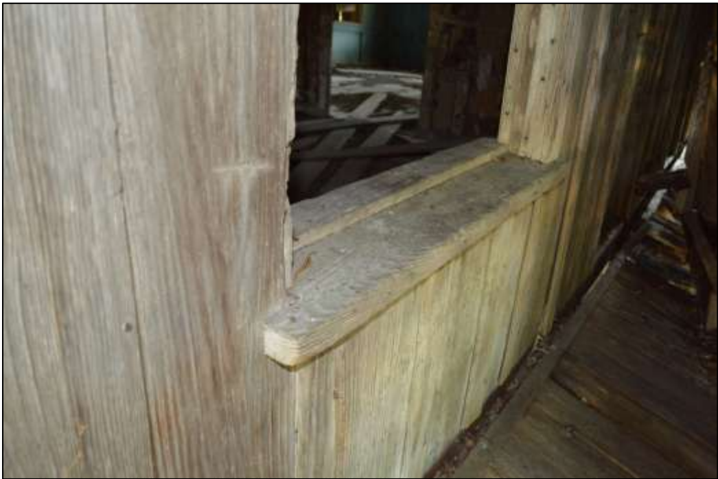
29. Window sills, jambs, and rail guards on south façade
