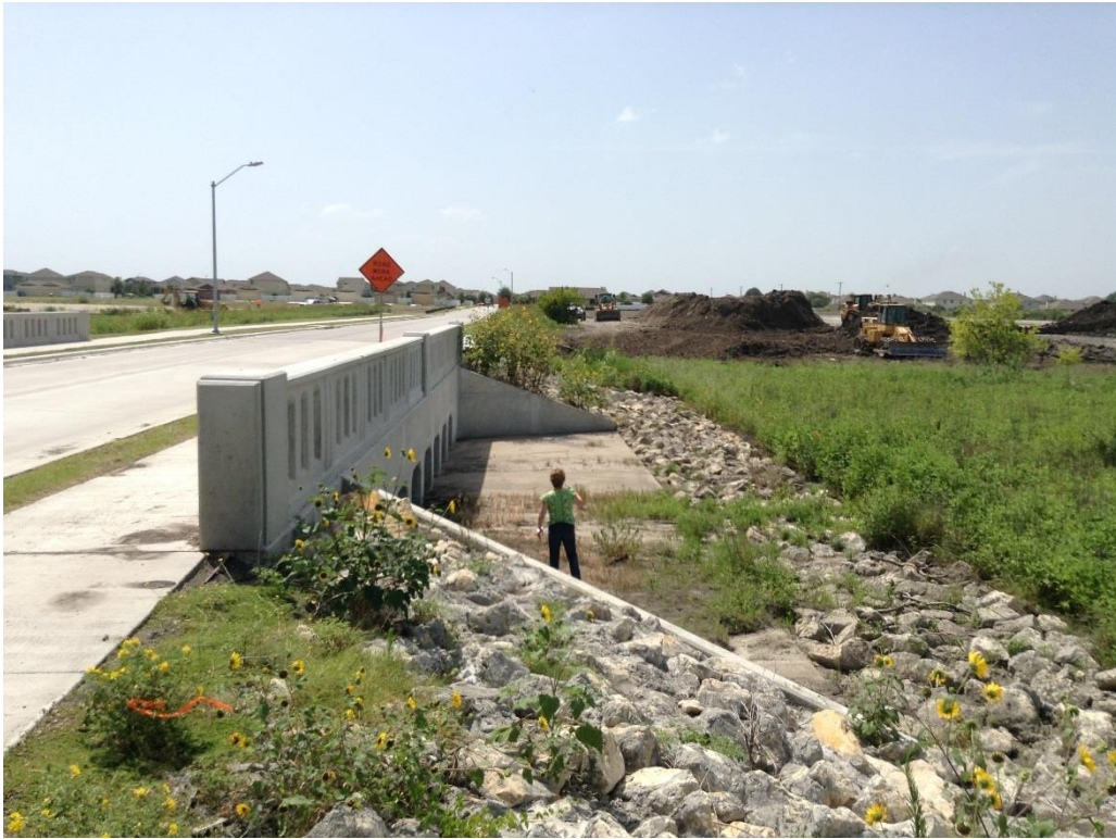
Photo 3: North side of culvert crossing at Town Center Drive, facing west. Tributary does not contain water at this location.
