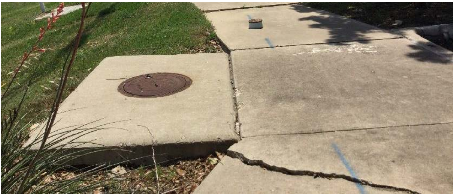
Figure 3-6: Cracked Sidewalk and Raised Water Valve
