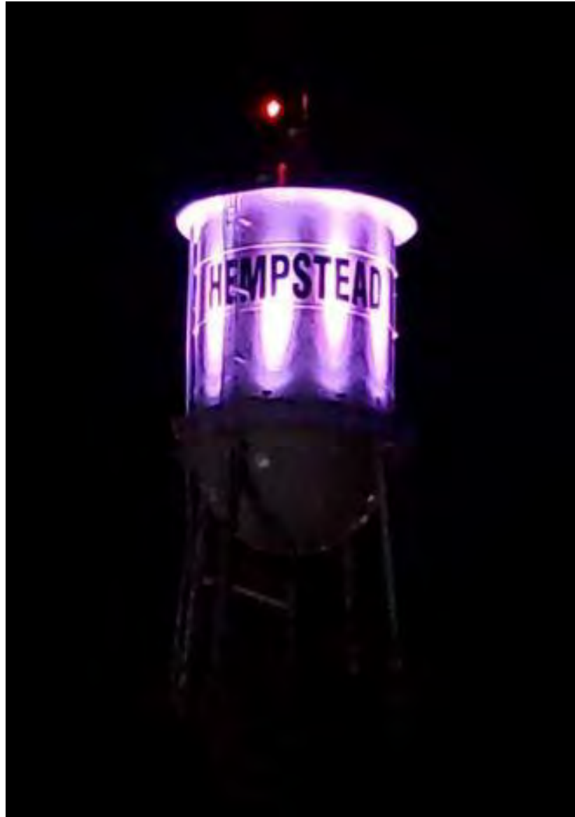
Alternate Bid Item #1 (10 lights on catwalk)
