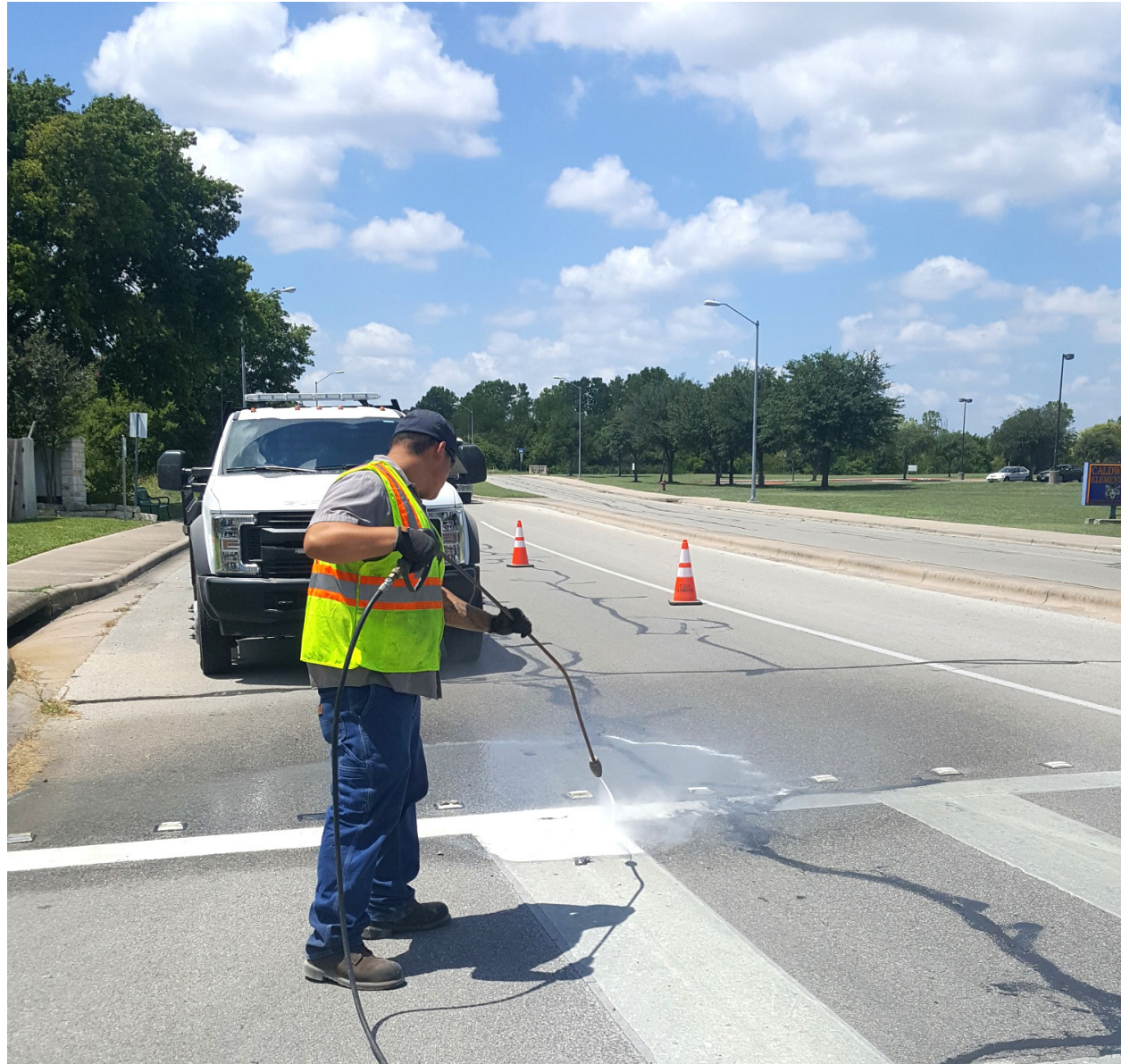
Crosswalk repairs in a Pflugerville neighborhood. Proactive maintenance extends the life of transportation infrastructure, improves safety and increases the comfort for road users for all transportation modes.
