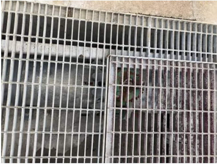
1. BUTTERFLY VALVE AND FLANGE ADAPTER ON 10" SS AIR HEADER
