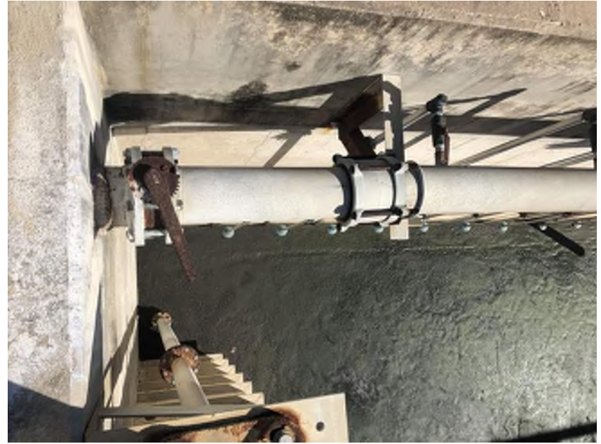
2. BUTTERFLY VALVE AND FLEXIBLE EXPANSION COUPLING ON 6" SS AIR HEADER
