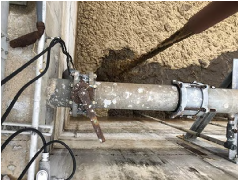
3. BUTTERFLY VALVE AND FLEXIBLE EXPANSION COUPLING ON 6" SS AIR HEADER
