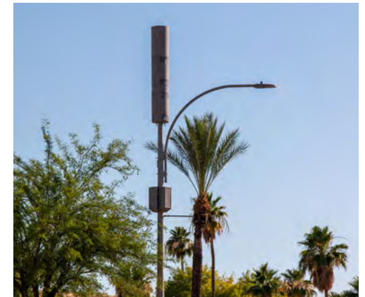
5G antenna on light pole
