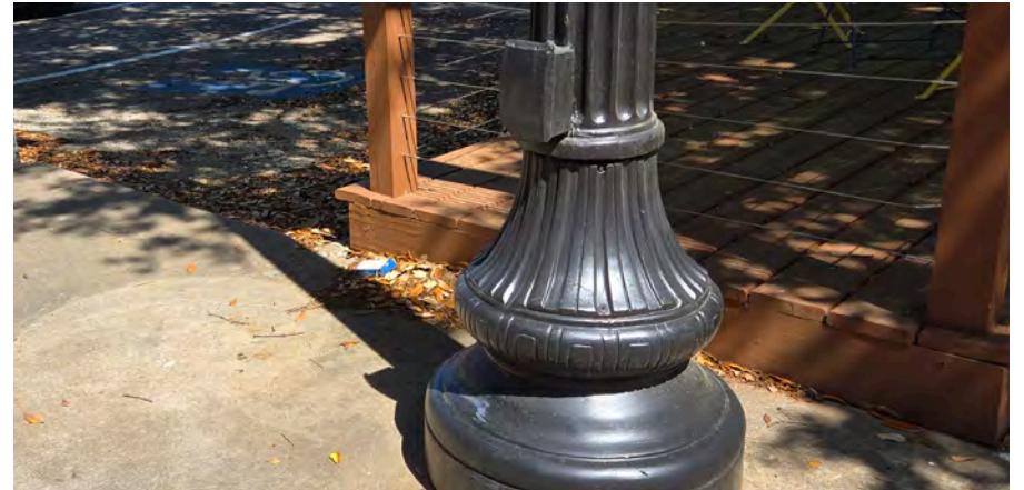
Fluted light pole bases with power receptacles
