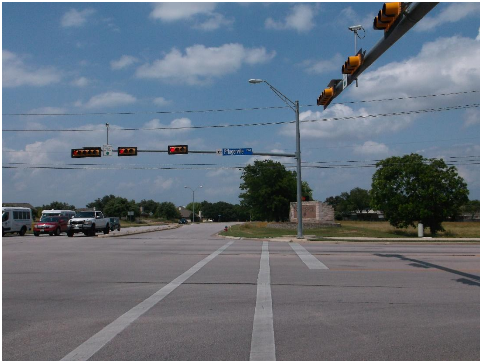
NB approach on Heatherwilde. Needs 4-section Flashing Yellow Arrow left-turn signal.
