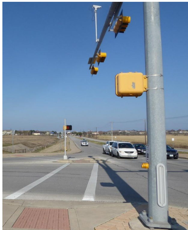
NE Corner – Ped-head not working
