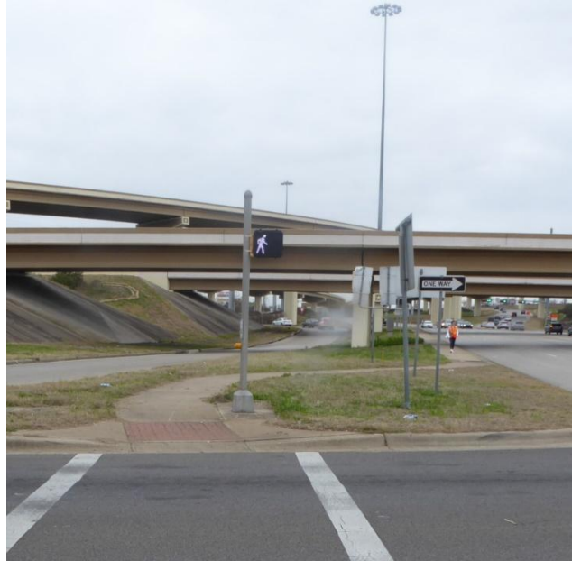
SE Corner – Ped push-button head not working for south crossing
