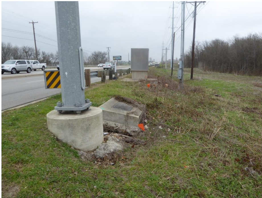
NE Corner – Existing ground box below ground surface exposed due to water scouring
