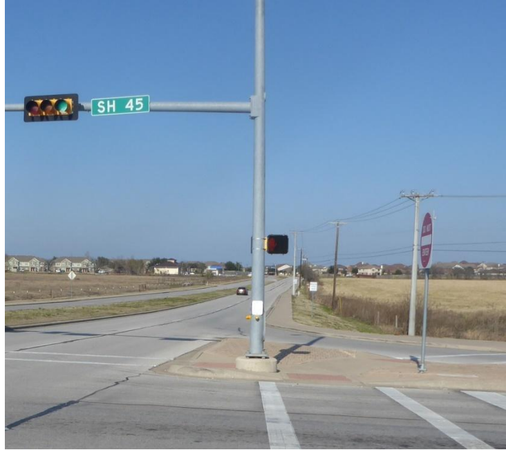
SE Corner – Ped-head not working
