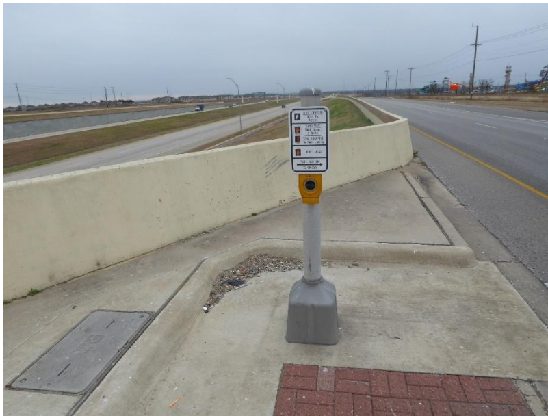
SW Corner – Ped push-button head not working for south crossing
