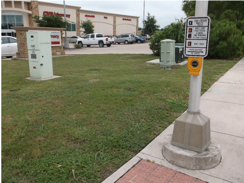
SW corner ramp is too short
