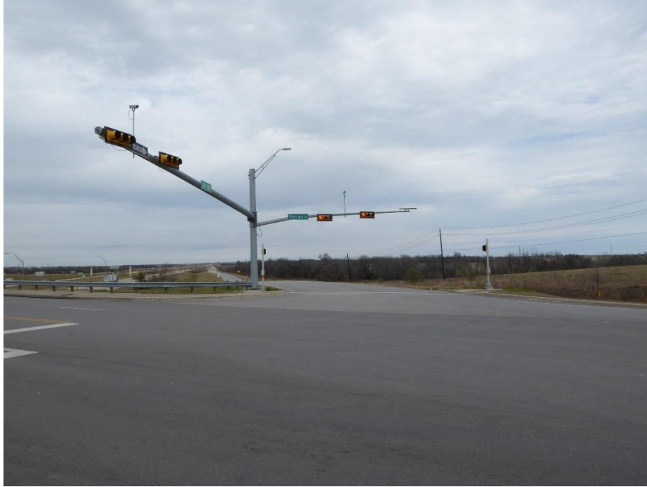
NB Approach – Mast-arm shaking vigorously in wind
