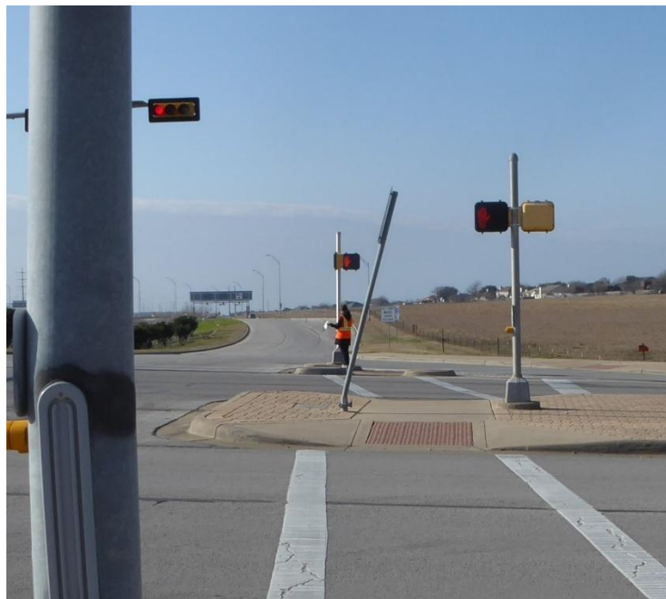
Ground mounted sign in NB median is bent
