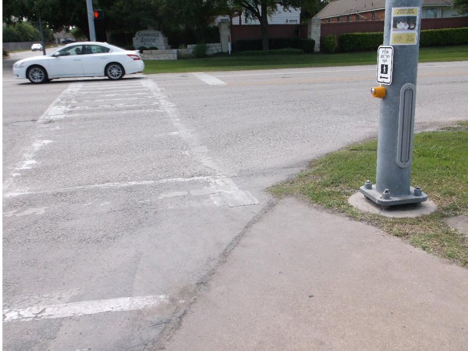
Faded crosswalk across SB approach
