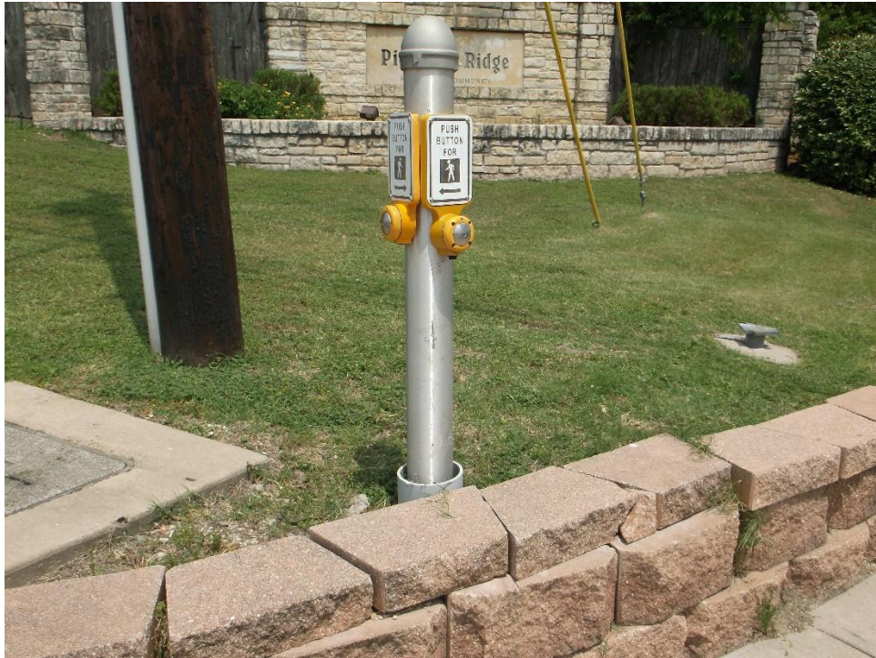
All pedestrian push buttons, including this one on the NE corner, are too far from the pedestrian ramps
