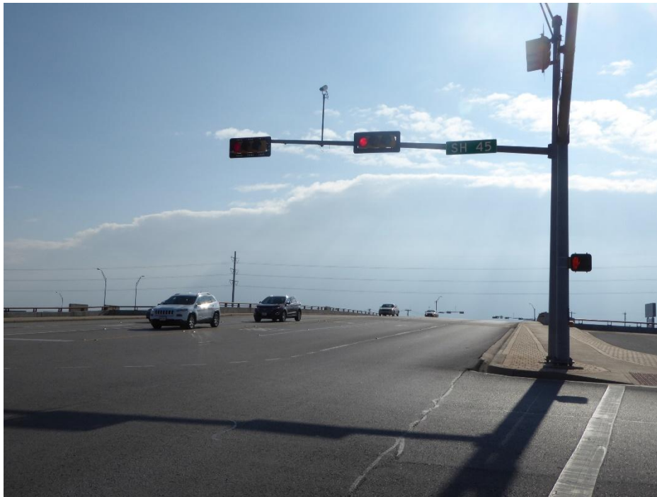
NW Corner – Ped-head is not working; Push-button beep not working
