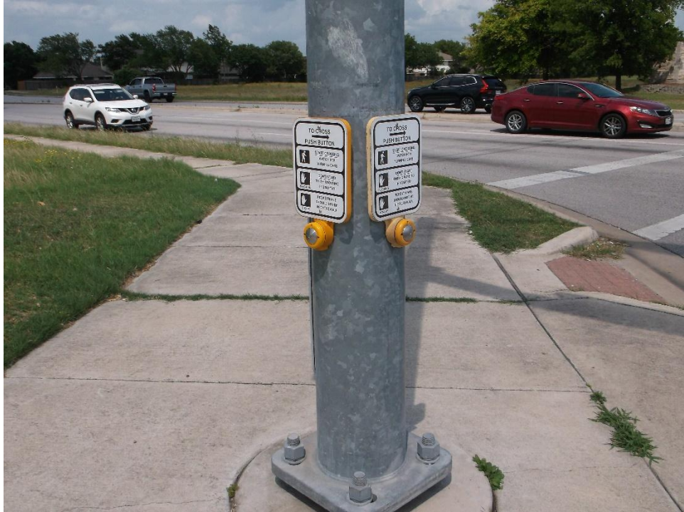
Pedestrian push buttons on NE corner are too quiet
