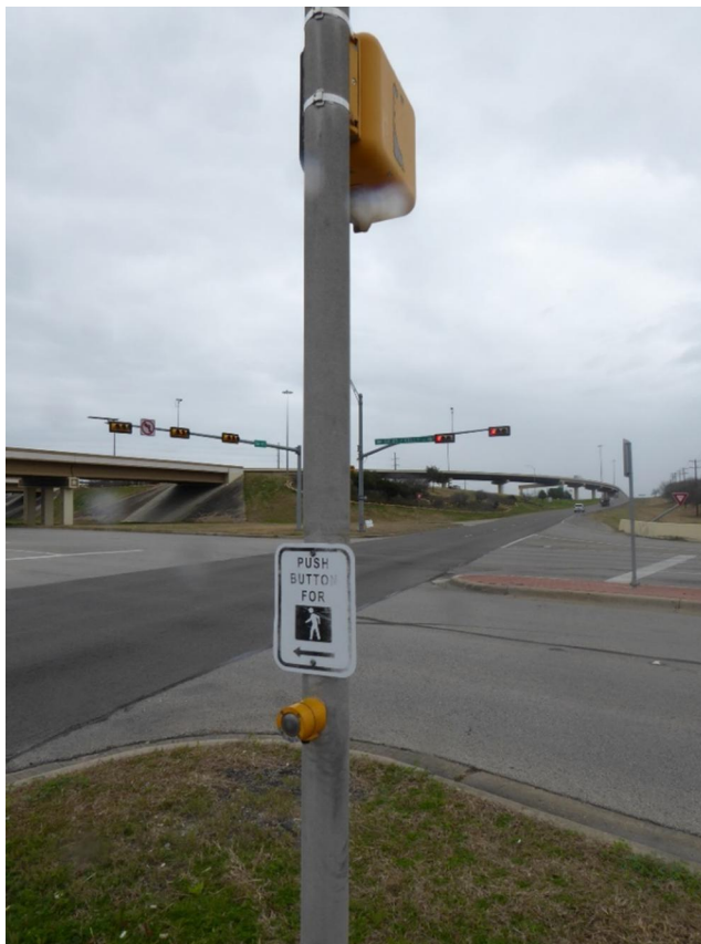
SE Corner – Ped push-button head not working for south crossing
