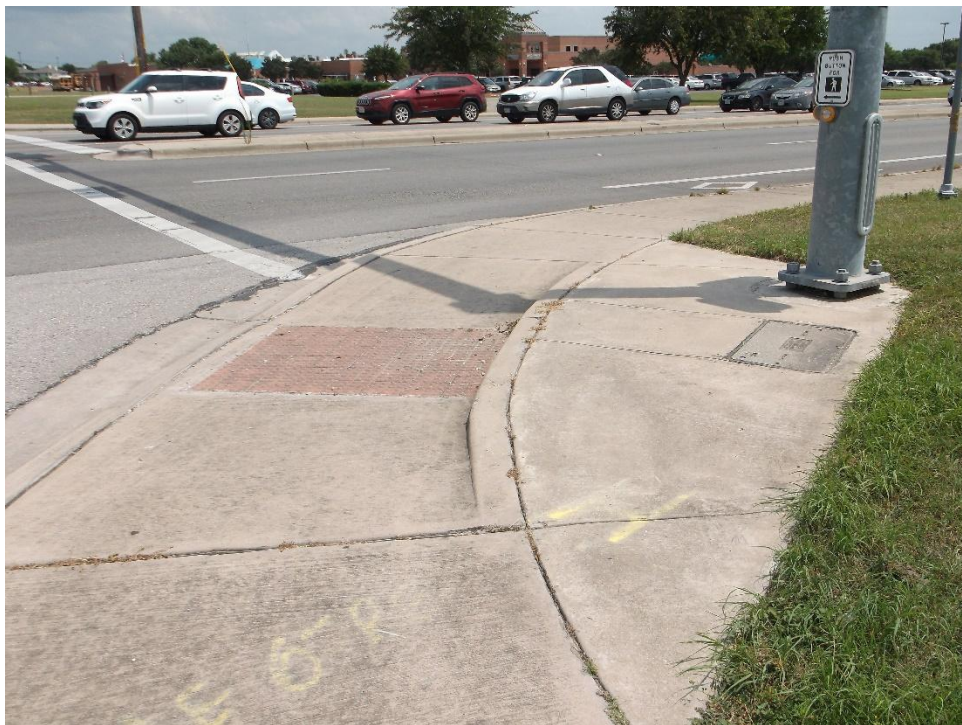
All pedestrian push buttons, including this one on the SW corner, are too far from the pedestrian ramps
