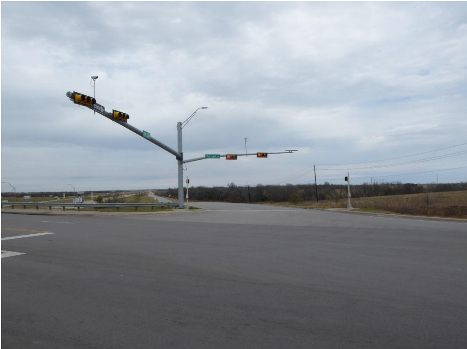
NB Approach – Mast-arm shaking vigorously in wind
