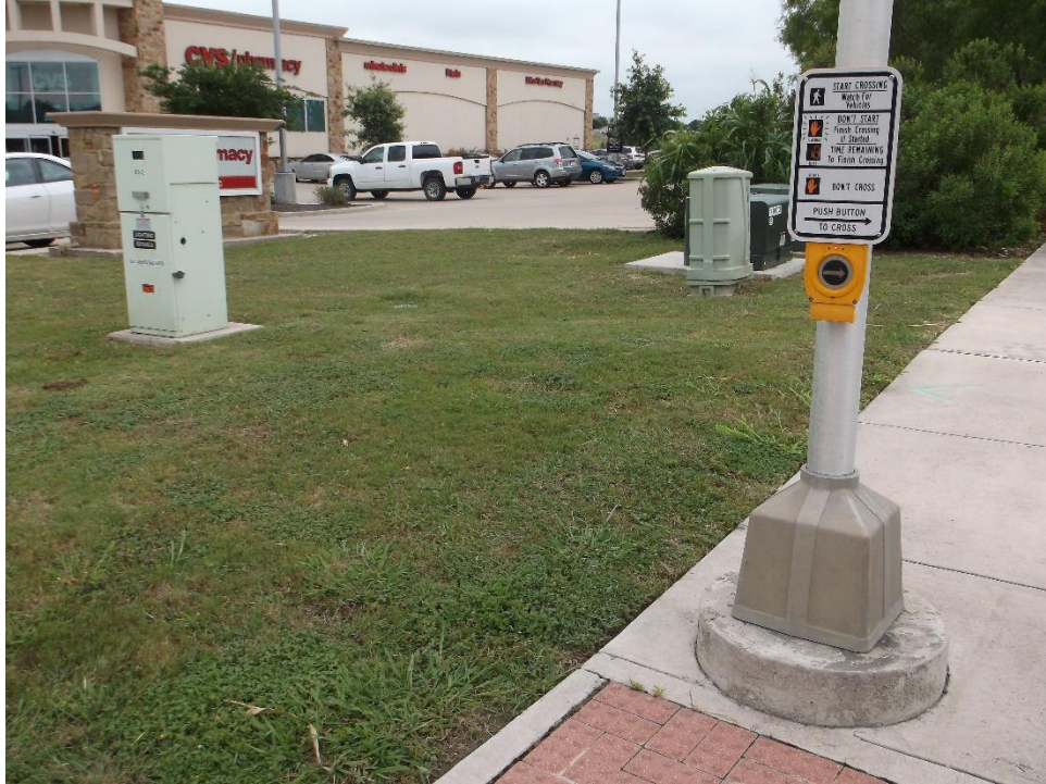
SW corner ramp is too short
