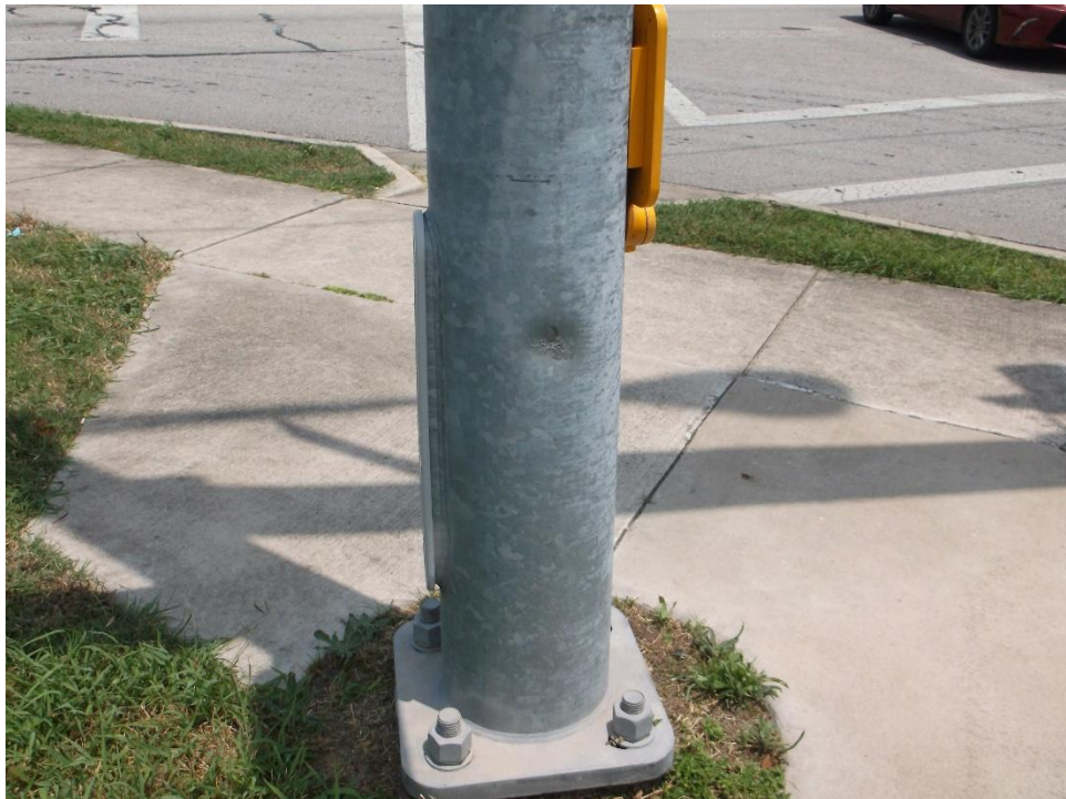
Dented signal pole on NE corner
