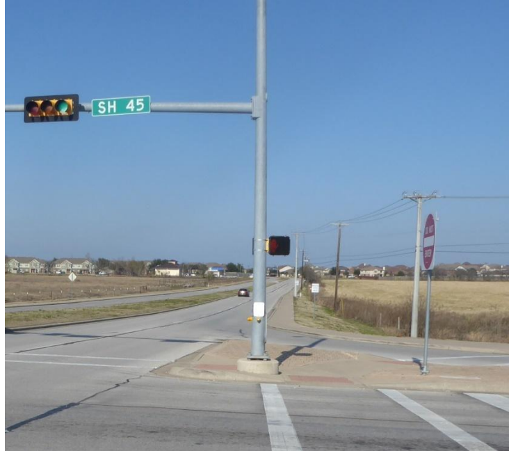
SE Corner – Ped-head not working
