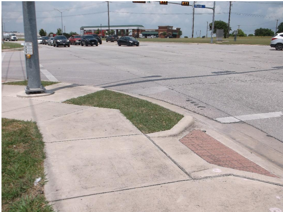
Pedestrian push button too far from ramp on SE corner
