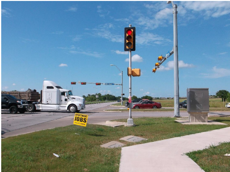
SE corner – pedestrian push button not accessible from sidewalk
