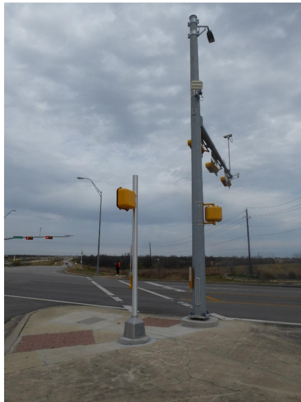
NE Corner – Ped push-button head not working for north-crossing
