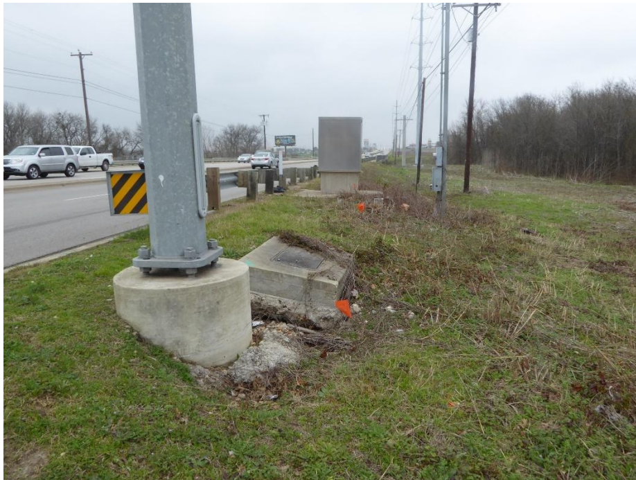
NE Corner – Existing ground box below ground surface exposed due to water scouring
