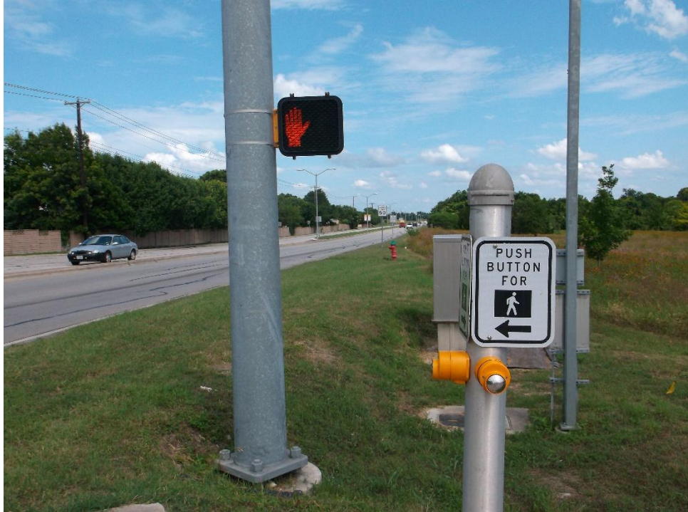
Pedestrian push button on SW corner
