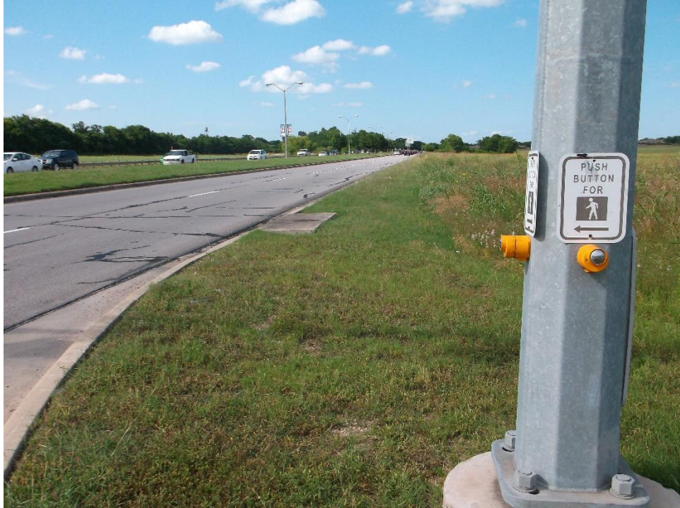
NE corner – pedestrian push buttons do not work
