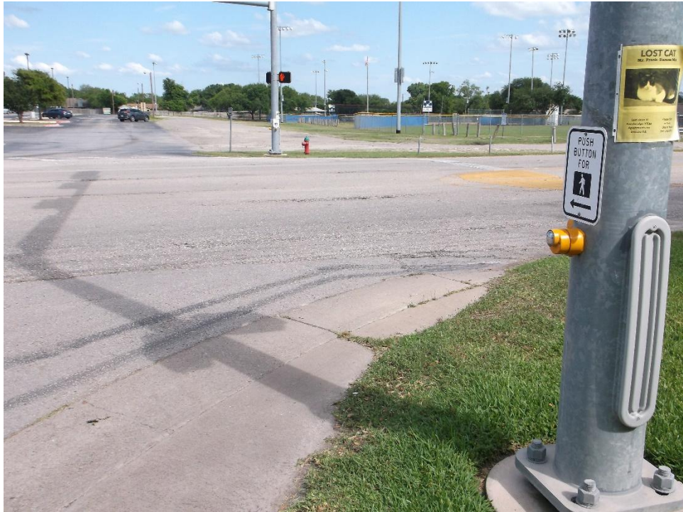
No sidewalk across NB approach
