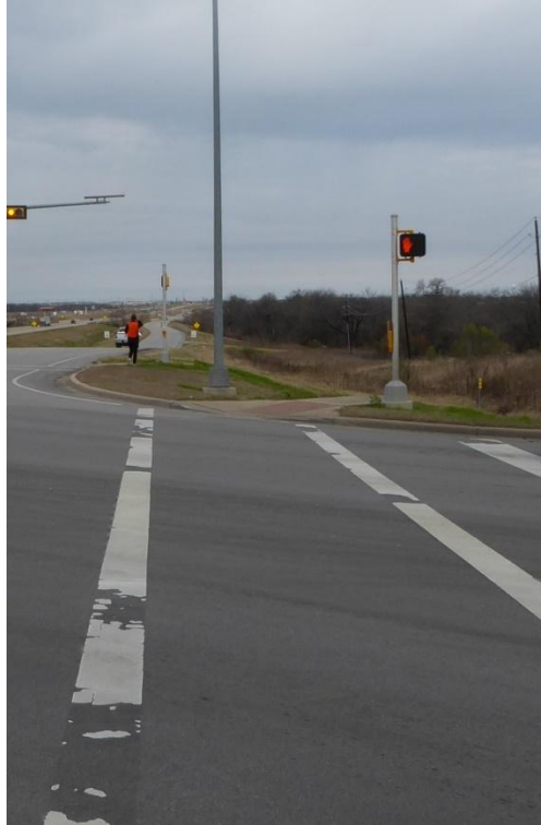
NW Corner – Ped push-button head not working for north crossing
