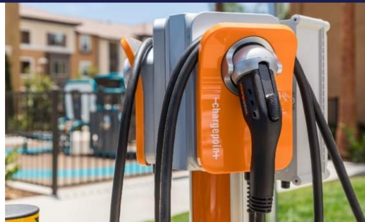
On-Site Electric Car Charging Stations
