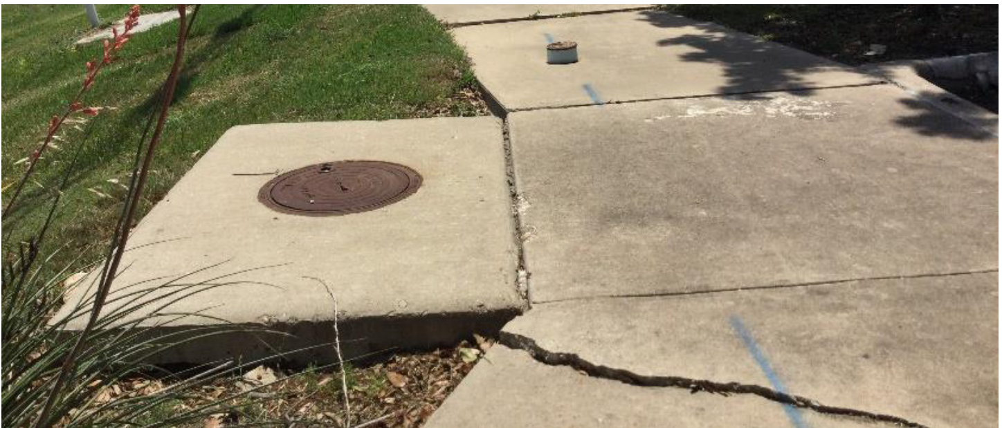
Figure 3-6: Cracked Sidewalk and Raised Water Valve
