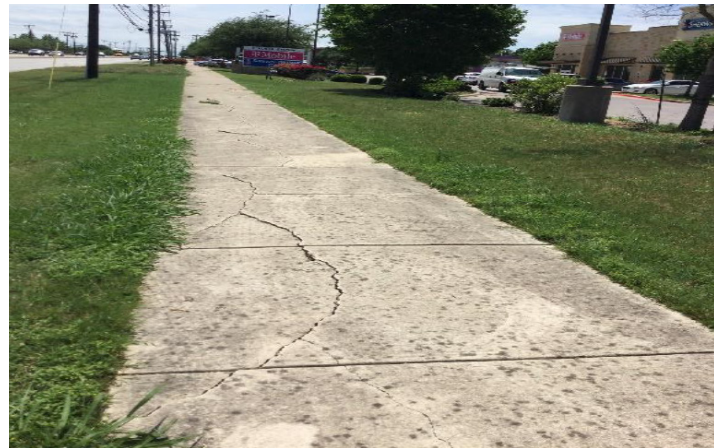
Figure 3-14: Cracked Uneven Sidewalks along FM 685
